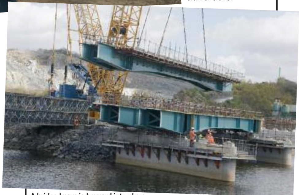
A bridge beam is lowered into place. Visible on the left of the picture is the temporary Bailey Bridge
